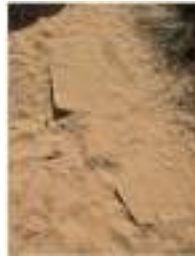
Evidence of prior better surface
